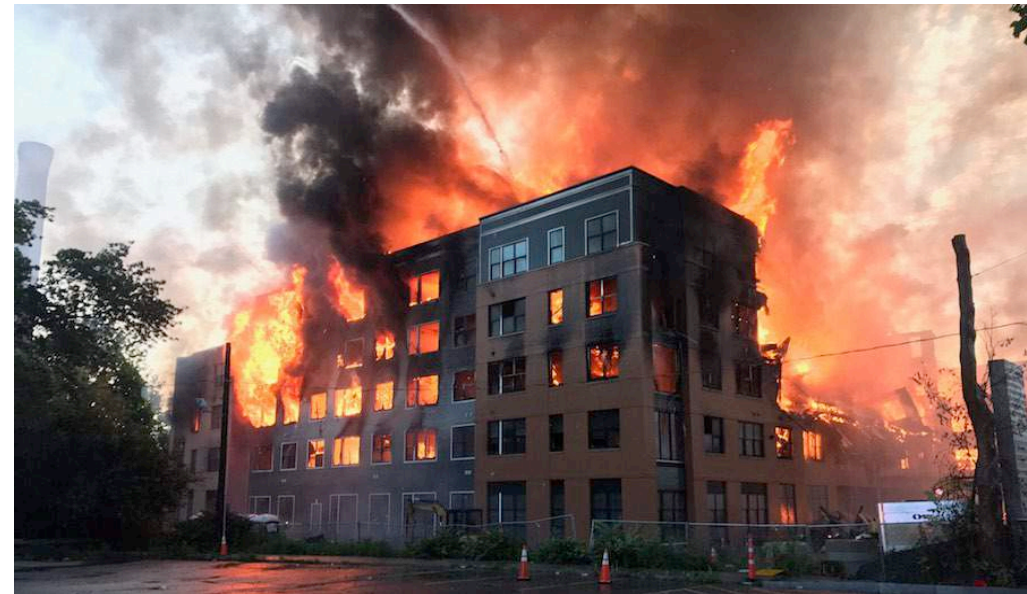
Fire in Timber Frame Apartment Building Under Construction (Source: Captain John Bonadio, Waltham Fire Department, as published at https://www.enr.com/articles/42484-what-local-officials-want-to-do-about-wood-frame-building-fires-in-massachusetts ), Courtesy of Waltham, Massachusetts Fire Department)
